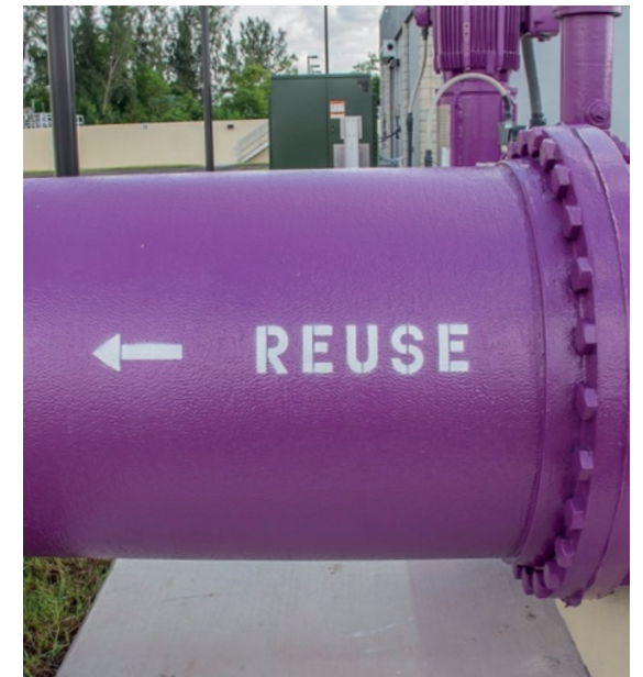
Purple pipes carrying reclaimed water in Florida
