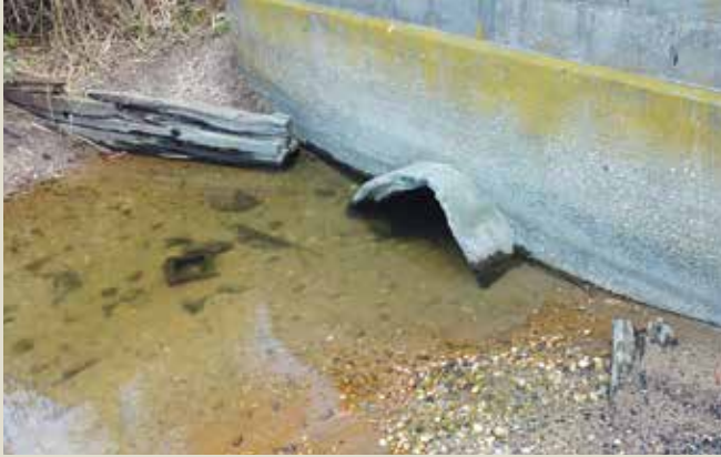
Undersized and perched culverts limit connectivity and restrict fish passage
